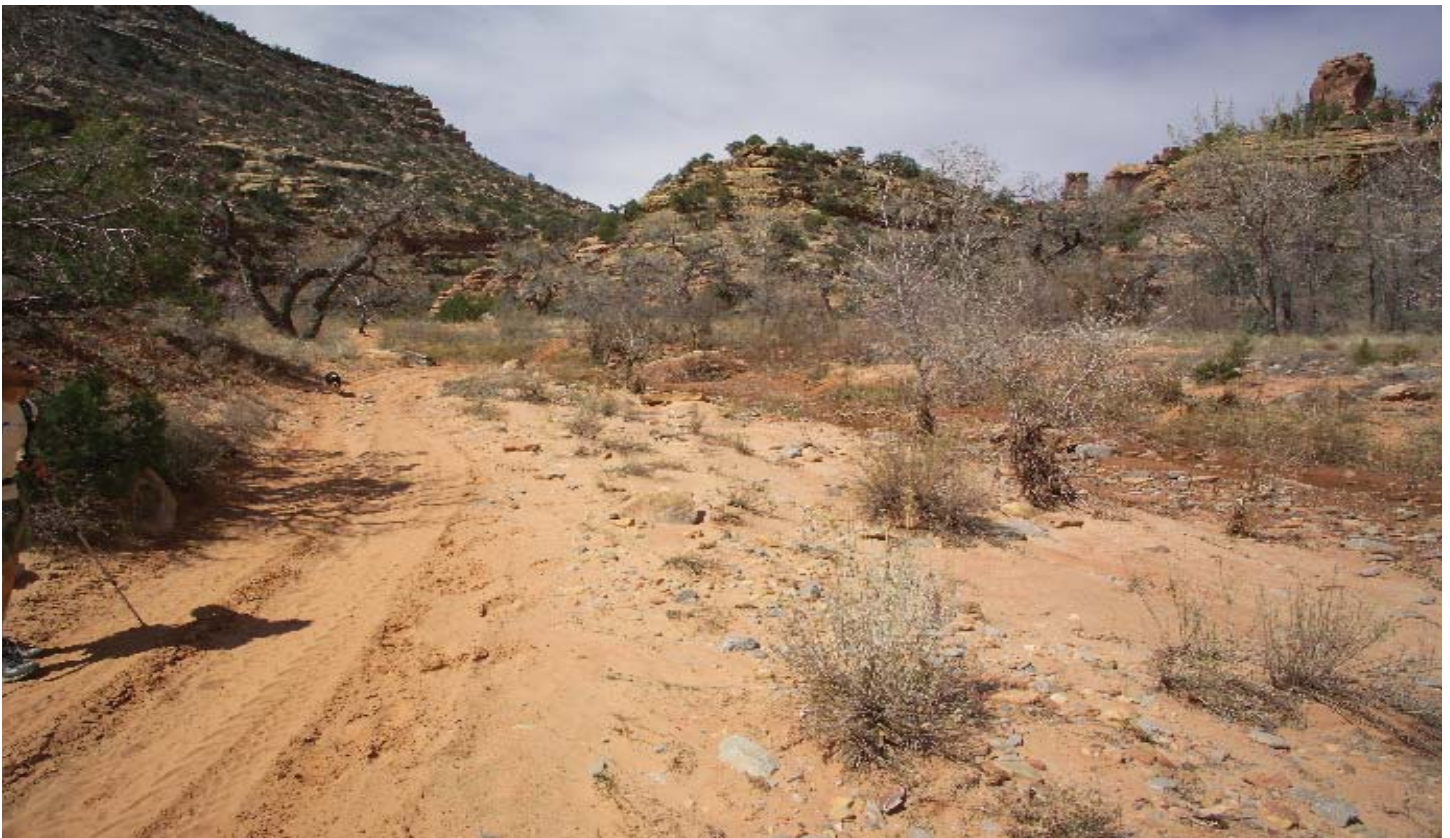
FIGURE 14. Area where high flows and lateral cutting of vegetation and soil scour the stream channel and floodplain, reducing shrub establishment and persistence. Arch Canyon, San Juan County, Utah.
