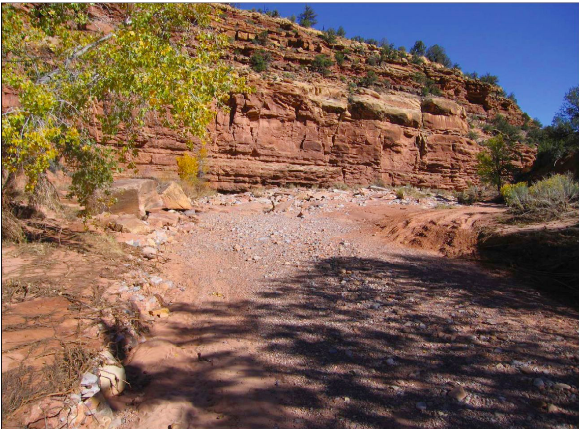
Figure 3b. Repeat photo of Figure 3a, taken in October 2006. Note the bank erosion and loss of vegetation along the bank on the left side and the exposed tree roots.
