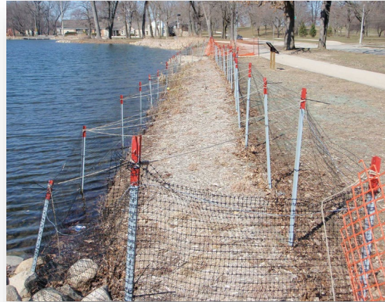
This temporary fencing will protect new, tall shoreline vegetation from geese until it becomes well-established
