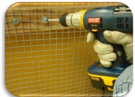
Attaching the mesh to the structure using an electric drill/driver, lath screws, and fender washers
