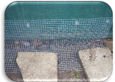
An "L" shaped apron of mesh with the bottom portion either buried or above ground will keep animals from getting under a shed
