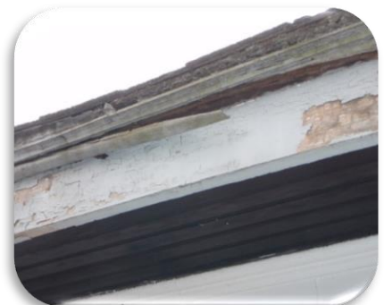
Rotten wood on this garage's fascia makes it relatively easy for animals to gnaw through. Repair or cover these areas with mesh to keep animals out
